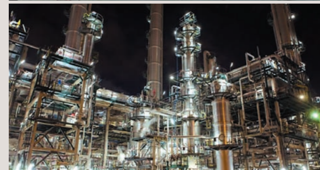
IOCL Gujarat Refinery
