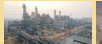
Left: Construction is proceeding on the 2nd stage. Right: Equipment installation work is starting. (Left and right pictures, as of Feb. 2014)
