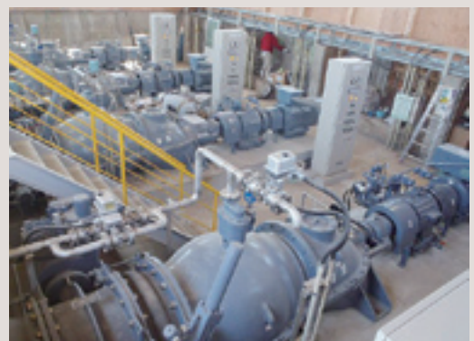
Donated drainage pumps (Pictured in front is the new pump no. 4)
