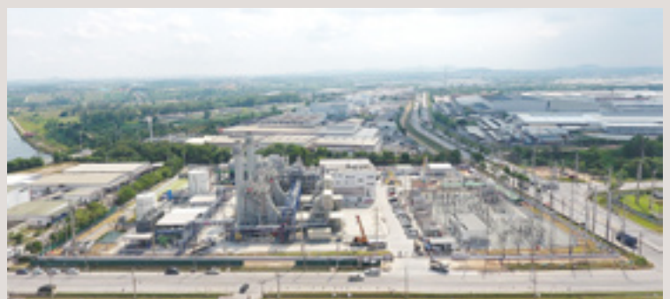
Plant No. 1, commencing operations in May 2017
