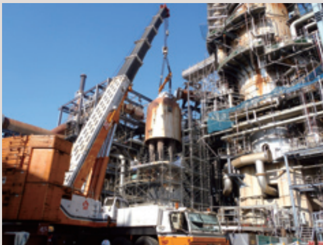
Plant during maintenance
