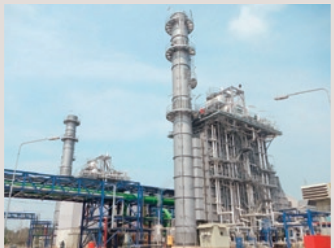
GKP1: the first completed plant in the project
