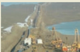
Natural gas pipe line in Azerbaijan (2002)
