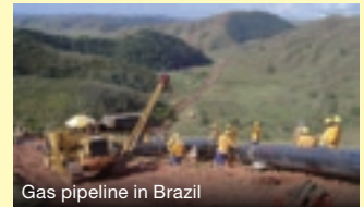
Gas pipeline in Brazil
