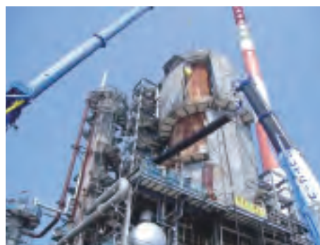
Client : Nippon Petroleum Refining Co., Ltd. Type : Turnaround for Fluid Catalytic Cracking Plant Location : Oita, Japan
