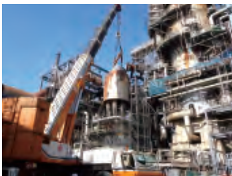
Client : Kyokuto Petroleum Industries, Ltd. Type : Scheduled Maintenance of Oil Refinery Location : Chiba, Japan
