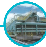
Japan Water Treatment Facility
