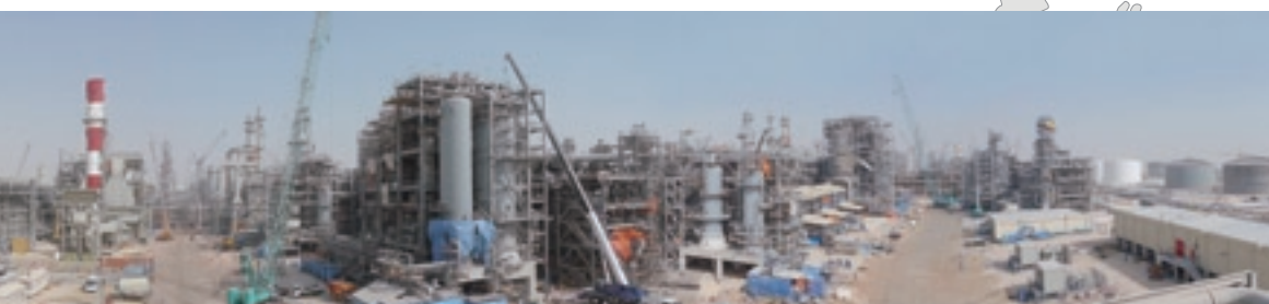
GTL liquid processing unit (Qatar)
