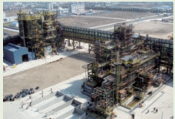
Siloxane project for Dow Corning Corporation in China
