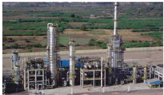
C2, C3, C4 Extraction Plant, Dahej - Client : ONGC
