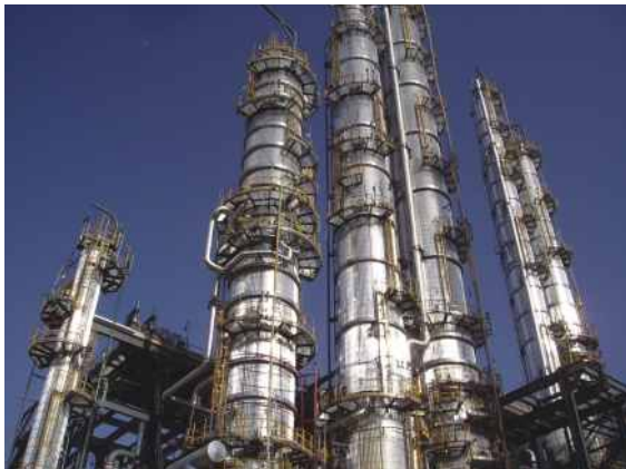
Butadiene Extraction Plant, Hazira - Client : RIL
