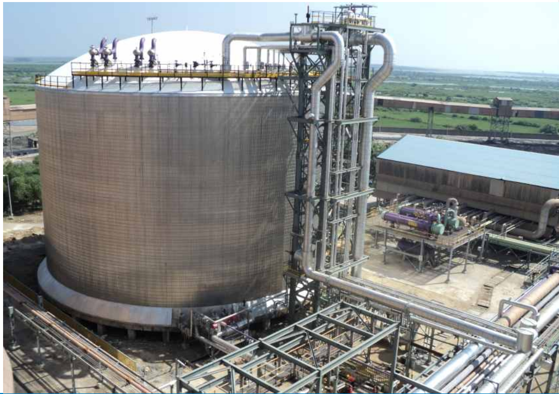
Ammonia Storage Facility, Paradip Client : IFFCO
